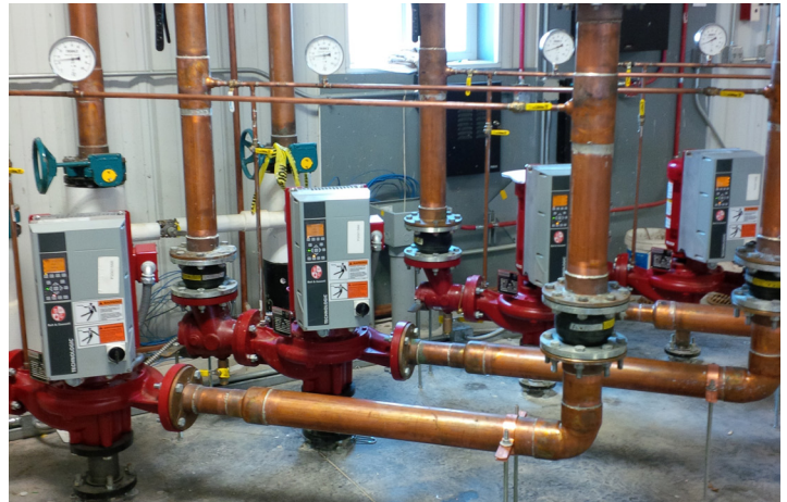
Series e-80 pumps installed with Technologic IPC variable frequency drive and Technologic PPS controller
